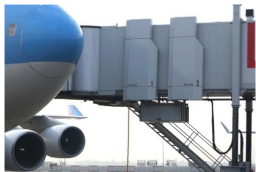
RAM402 retriever, installation on the side of the passenger bridge
