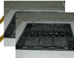
Ground pits, retractable pits and coilers
