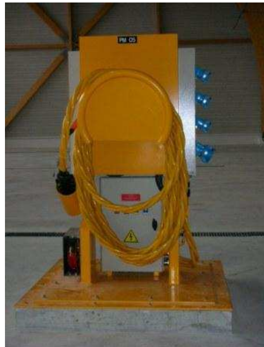
400 Hz cable on coiler
